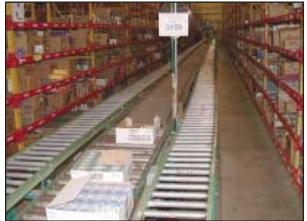
CONVEYORS AND RACKING
