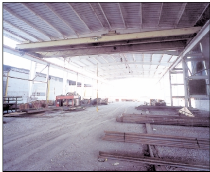
ROBBINS & MYERS 5-TON CAPACITY DOUBLE-GIRDER TOP-RUNNING TRAVELLING BRIDGE CRANE
